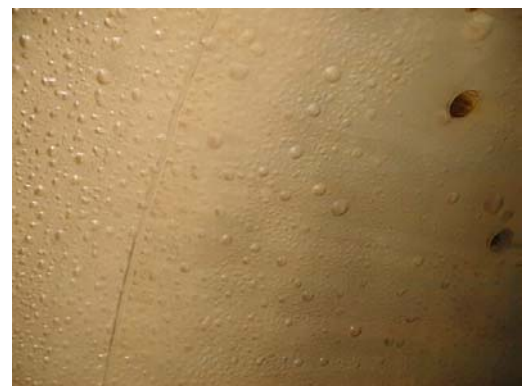
Example of Cold Wall Effect Blistering in a Steel Tank
