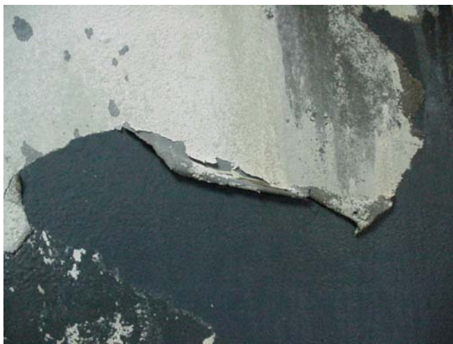
Figure 8: delamination of lining
